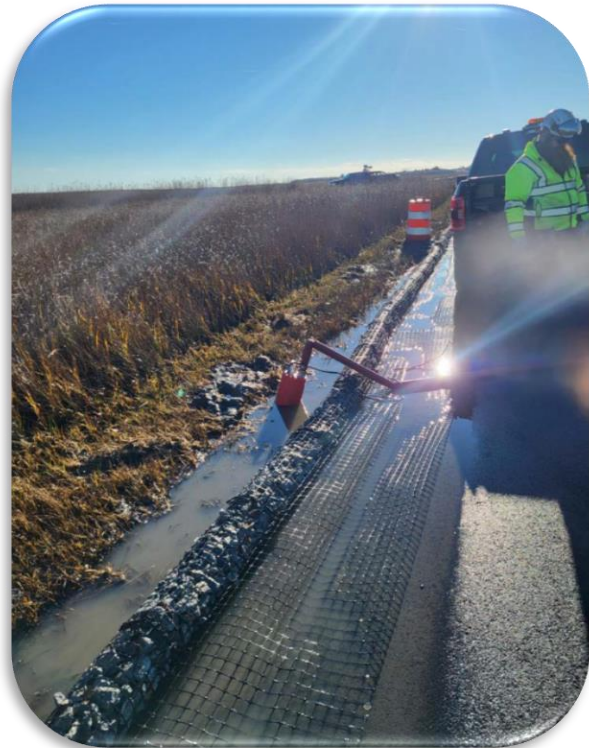
Figure 1111: Dewatering Efforts along South Bowers Road Prior to Paving Demonstrating High Water Levels Encountered
