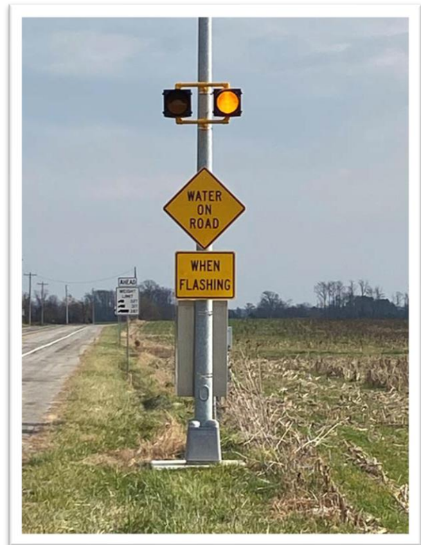
Figure 1414: "Water on Road" Warning Sign System
